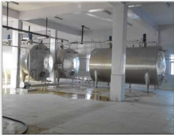
Horizontal Milk Storage Tank
