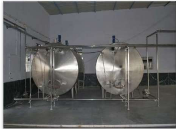
Horizontal Milk Storage Tank
